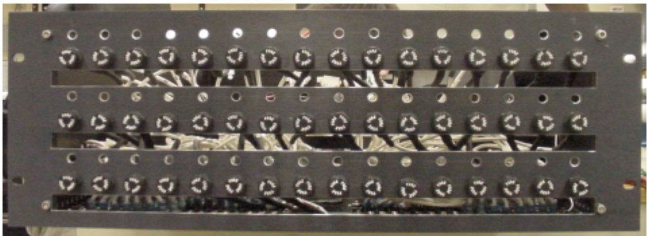
Figure 6-2 (Front Panel with 48 fuses)
