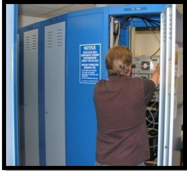
Working in Hall A&C Equipment Racks
