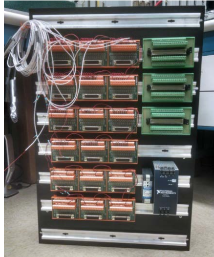
Slow controls patch panel
