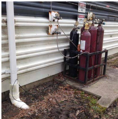
Flammable gas pad and lines.
