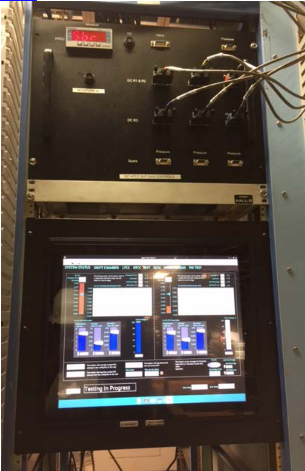
PID loop test: control panel
