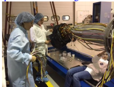
Mindy Leffel, Amanda Hoebel, Brian End, and Marc McMullen (not in picture) routing R1-R3 cables
