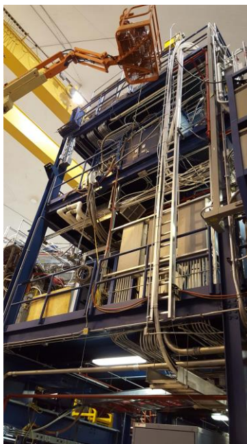
DC gas lines
