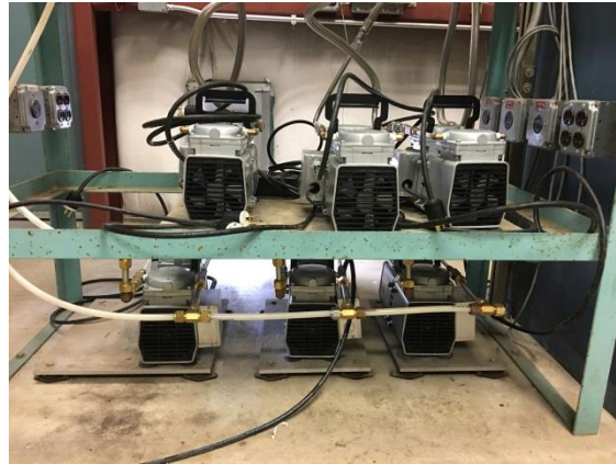
New DC gas return pumps, with fittings from old pumps.
