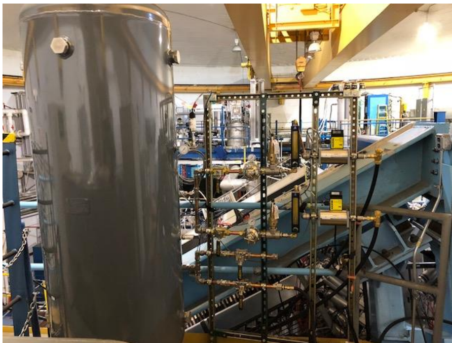
Air-cooling tank and panel on top deck of Forward Carriage.
