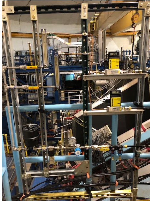
Nitrogen panel on top deck of Forward Carriage. Nitrogen flow set to ~20 L/min for each output, providing a total flow to RICH of ~40 L/min.
