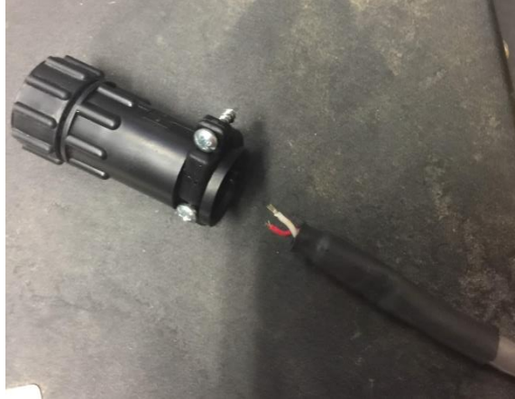
Broken output enable cable for SVT chiller pump's relay box.
