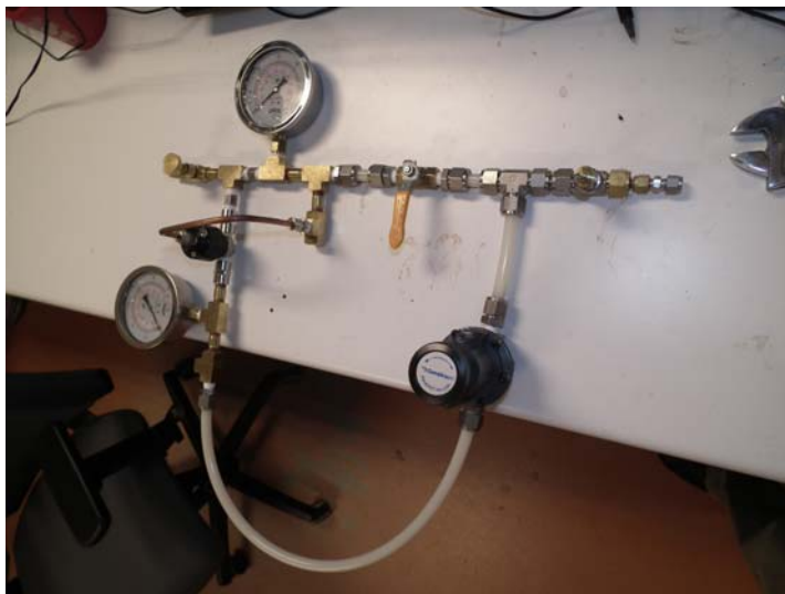
Figure shows some of the gas system components assembled for RICH N2 Auto-change
