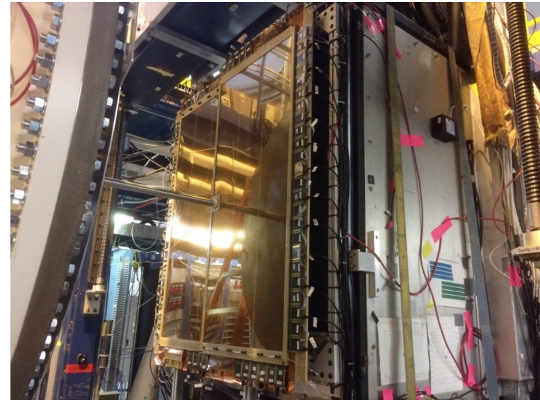
2 GEM detectors installed in Hall B beam line, May 2016
