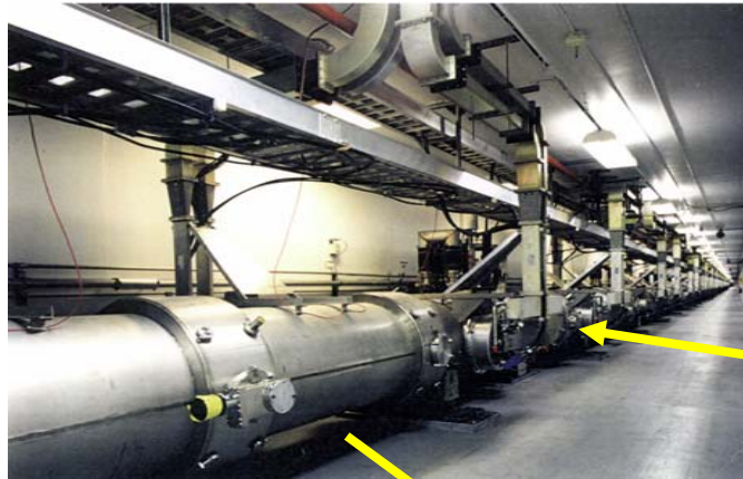
Cryomodules in the accelerator tunnel
