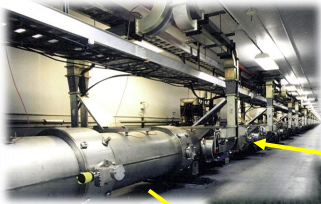
Cryomodules in the accelerator tunnel
