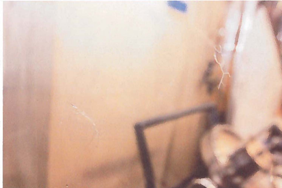
View of Double Walled Plastic Clean Area(s) Sheeting w/ Holes from Projected Glass
