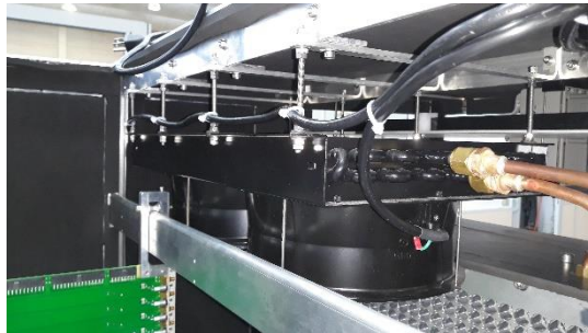
Top heat exchanger
