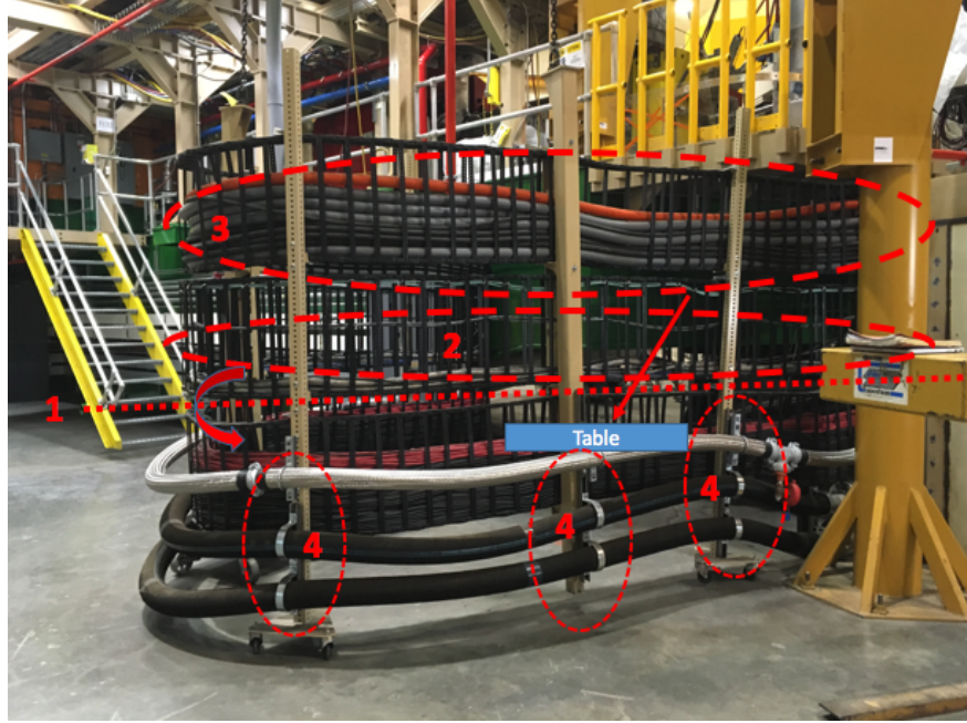
Figure 8: The SHMS cable tray showing the modification steps needed for LAD. 1: Cable tray support poles will be replaced and shortened. 2: The middle cable tray will be disassembled and secured to the lower tray. 3: The upper cable tray will disassembled and the cables will rest on a table near the pivot. 4: Support brackets will be installed on the support poles to carry the flexible hoses.
