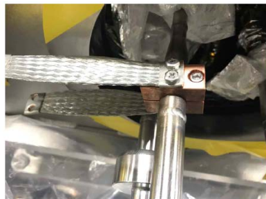
[Connect copper thermal braids to the pipe]
