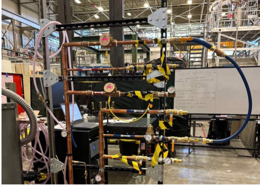
LCW Panel currently configured to test top MPS flowmeter
