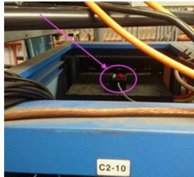
Deployed box circled in magenta
