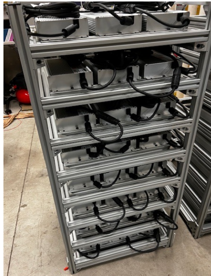
Rear view of rack
