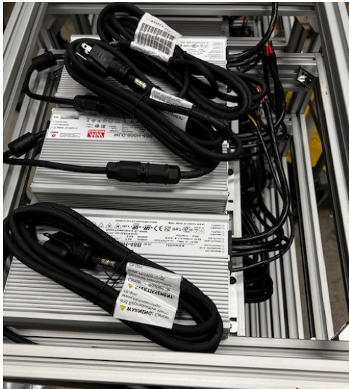
Top view of rack
