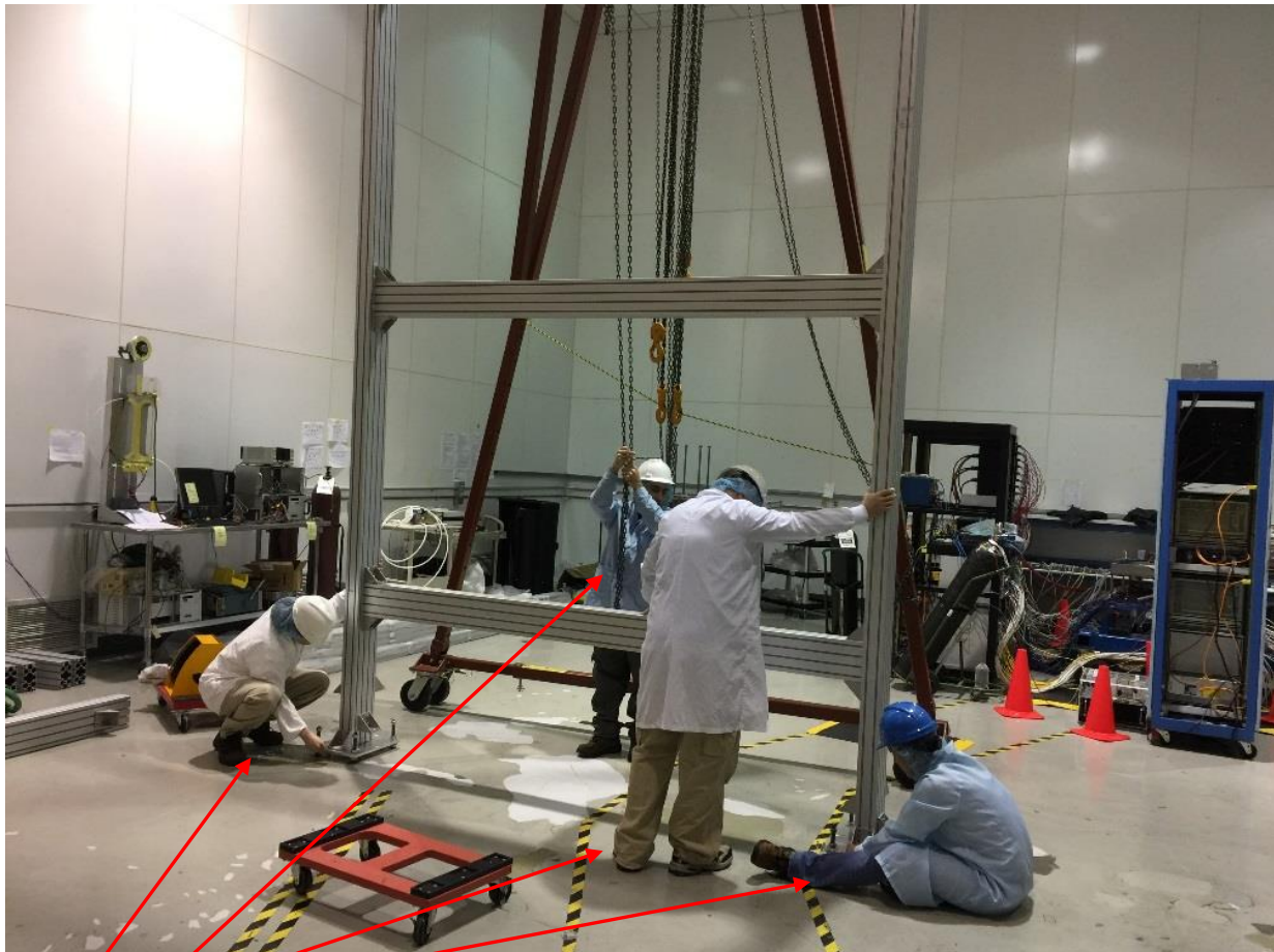
Brian, Sahin, George, and Mindy lifting right side of assembly structure to fasten it to anchored base plates.
