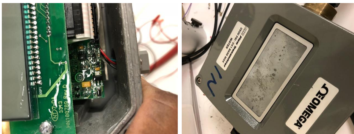
Photos of SVT "in" flowmeter showing evidence of internal moisture.
