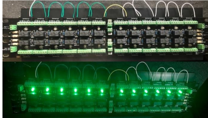
Testing the relay circuits of the SoLID Motor Controller PCB as a bus
